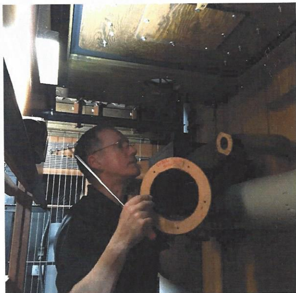
The wind supply is disconnected in preparing for removal of the Schwimmer.
